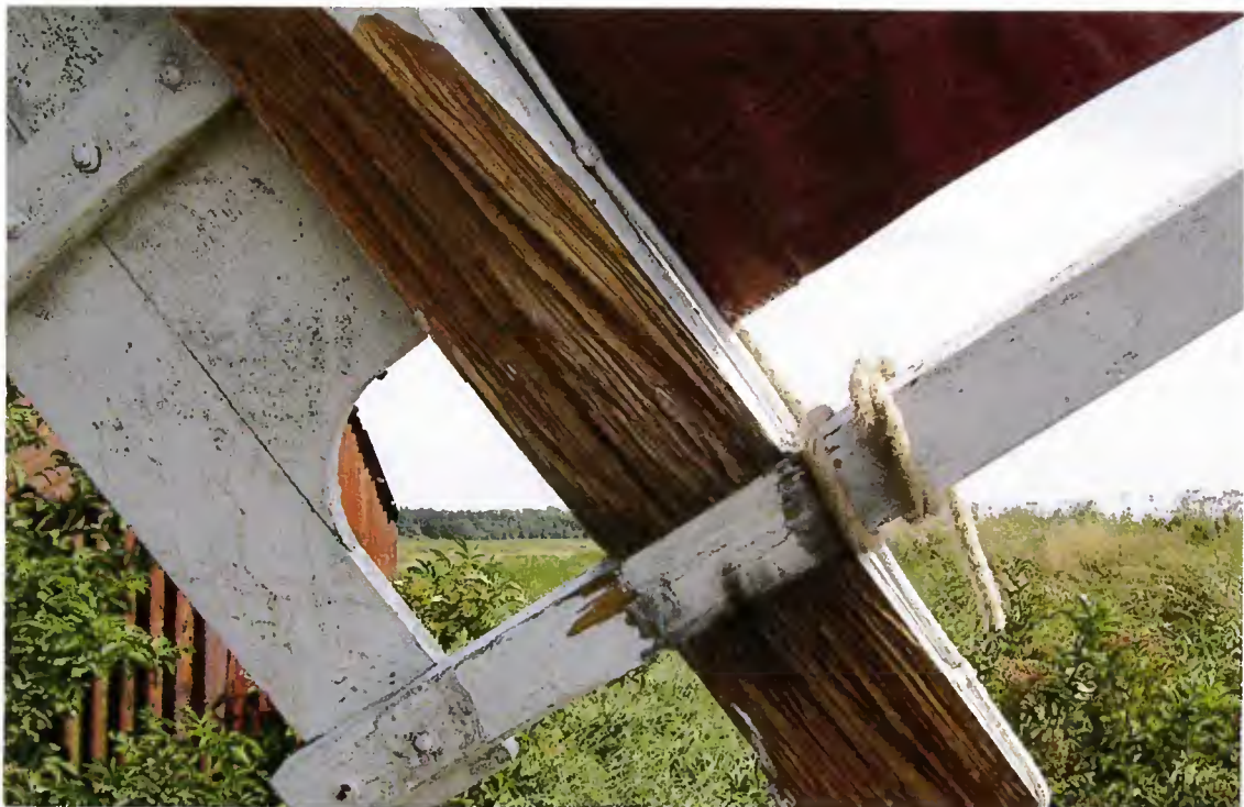
The damaged sail whip at Herringfleet
