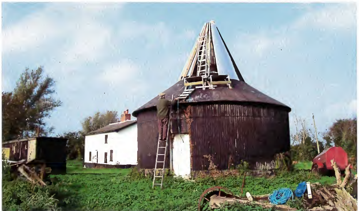
Chris Hullcoop returns to rig a temporary cover on Syleham mill for the winter - this time making sure the ladder is tied! (14th October)
