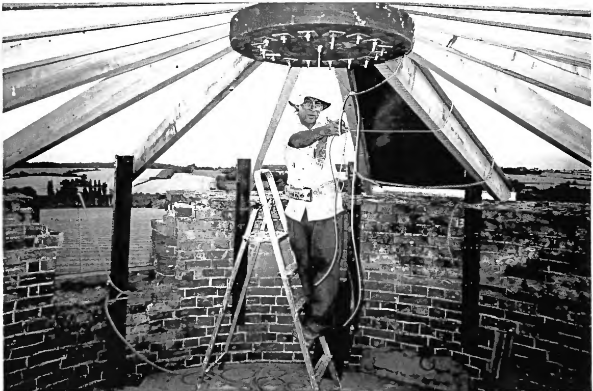
Chris Hullcoop preparing to fit the first aluminium sheet (Photo: Steve Binks)
