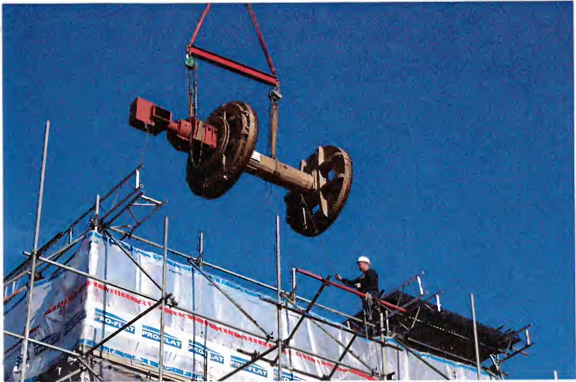
The repaired windshaft being lifted back into Drinkstone post mill on November 1st 2005
