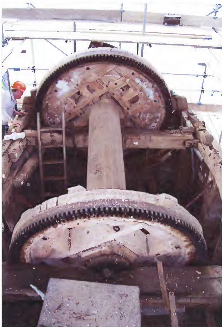
View from the top of the scaffold on June 9th showing the windshaft assembly ready to be lifted out.
