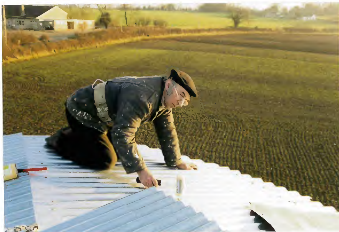
Chris Hullcoop working on the new roof at Great Whelnetham mill (February 1997).
