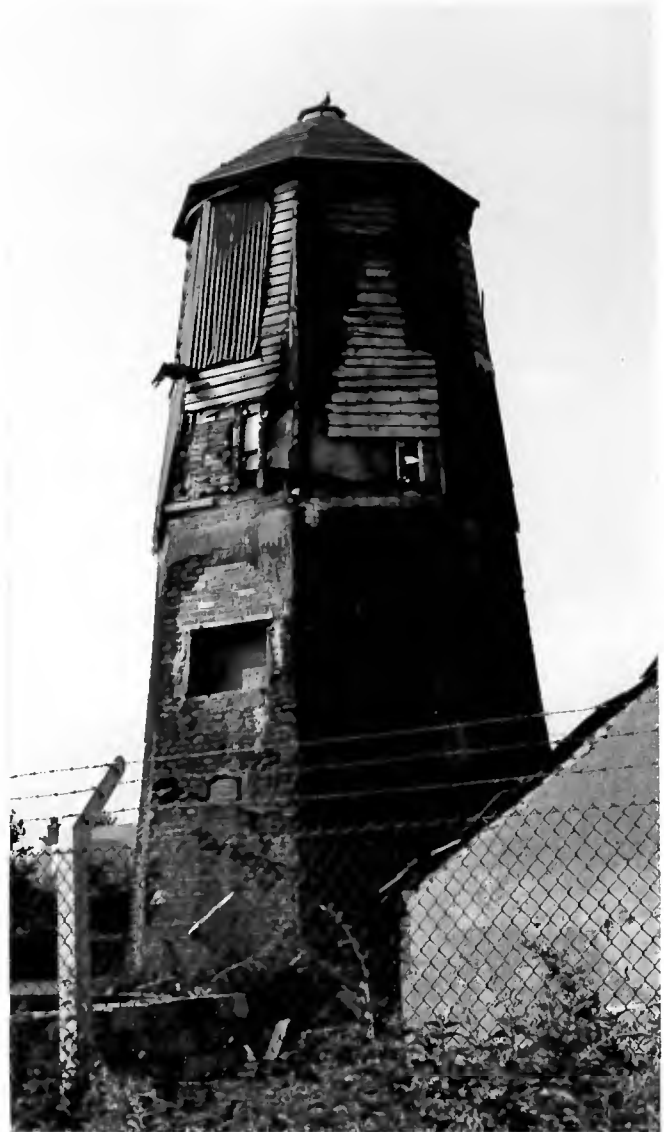
Walton mill after the fire, showing badly charred cant post & boarding
