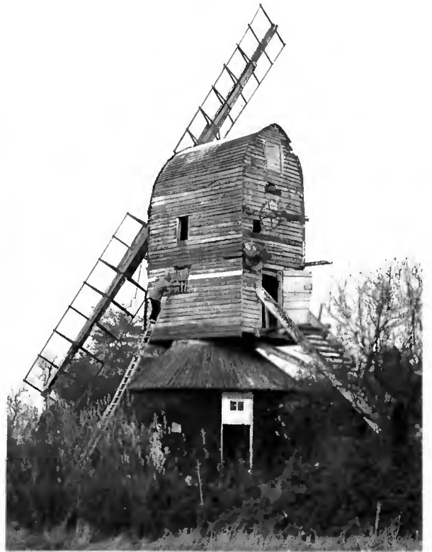
Above: Mark Barnard working on the weatherproofing of the buck windows. (Photo: Chris Hullcoop)
