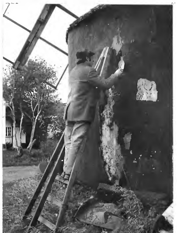
Below: Chris Hullcoop patching up the rendering on the roundhouse. (Photo: Mark Barnard)
